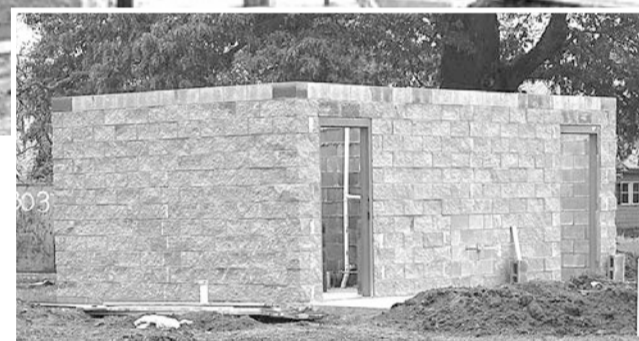
By Mayor Myron Mixon - Citizens of Unadilla, the new Splash Pad restrooms are coming along. The walls are complete on the restrooms. We are getting closer and closer to opening. I know the kids can't wait to get wet this summer.
